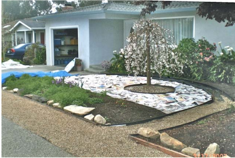
Second area, covered with newspaper, ready for mounded dirt. It will form a swale in front yard to catch rain water.
